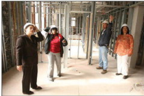
CR Staff/Owen Sweeney III Jim Vincent (center right), site manager for Serenity Place, gives Marian House residents Danielle McPhearson (left), Willette Fair and Mia Smith a tour of the construction site. Serenity Place will open in September 2007 in the former Holy Spirit School, Baltimore and will house 15 single and four family apartments.
